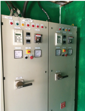
STS Control and Monitoring Panel
