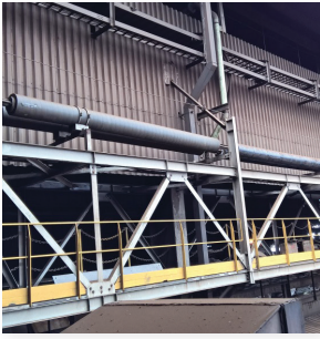
Pre-insulated Piping and Thermally Isolated Pipe Supports for the 2 Parallel Pipelines
